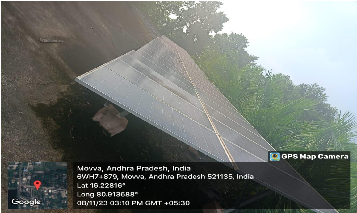
Solar Panels Placed on the roof of the college
