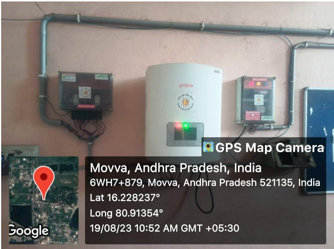
Solar Panels Grid link Placed in the college opposite to the principals chamber.
