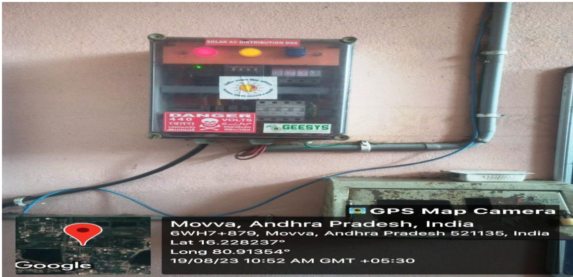
Solar Junction Box Placed in the college opposite to the principals chamber.
