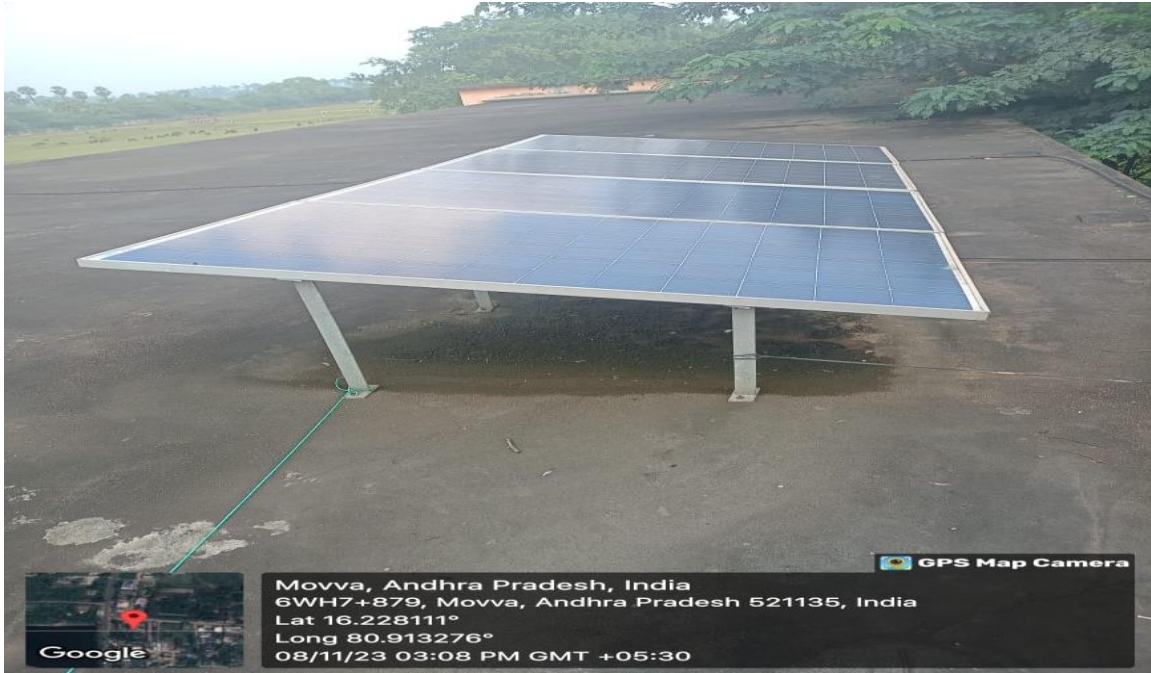
Solar Panels Placed on the roof of the college
